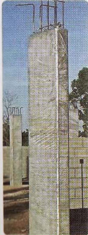
Plastic wrapped around a concrete column
