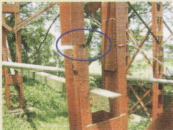
Faulty column connection
